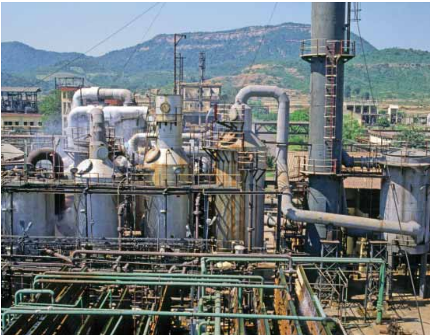
VANGUARD OF GROWTH STORY: Prospects for the heavy engineering industry have brightened in recent years
